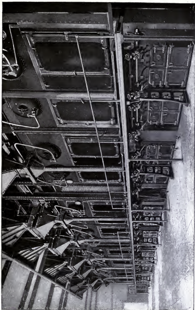
VIEW OF 4000 H. P. OF BOILERS AND RONEY STOKERS Installed in Plant of the Edison Illuminating Company, Boston, Mass.
